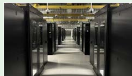
▲ The energy efficiency management of lighting systems was implemented by the Shanghai free trade zone machine room. (Photo provided by the Data Center)
