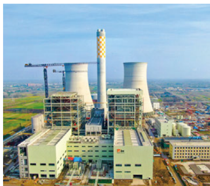
ABC Hubei Branch actively supports the clean and efficient use of coal. (Photo credit: ABC Hubei Branch)
